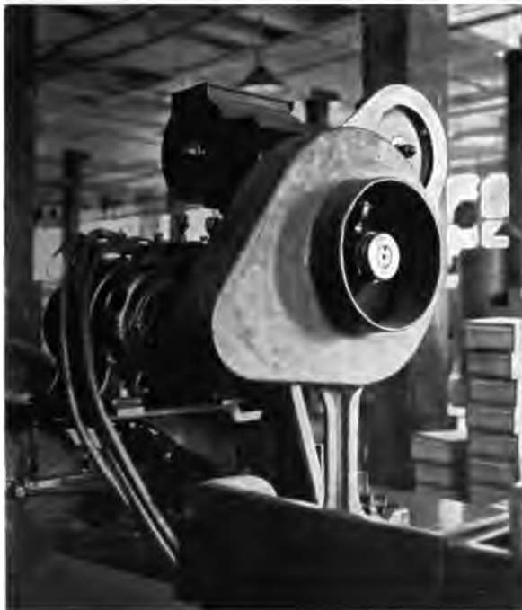
Fig. 3. Protected individual Motor Drive.
